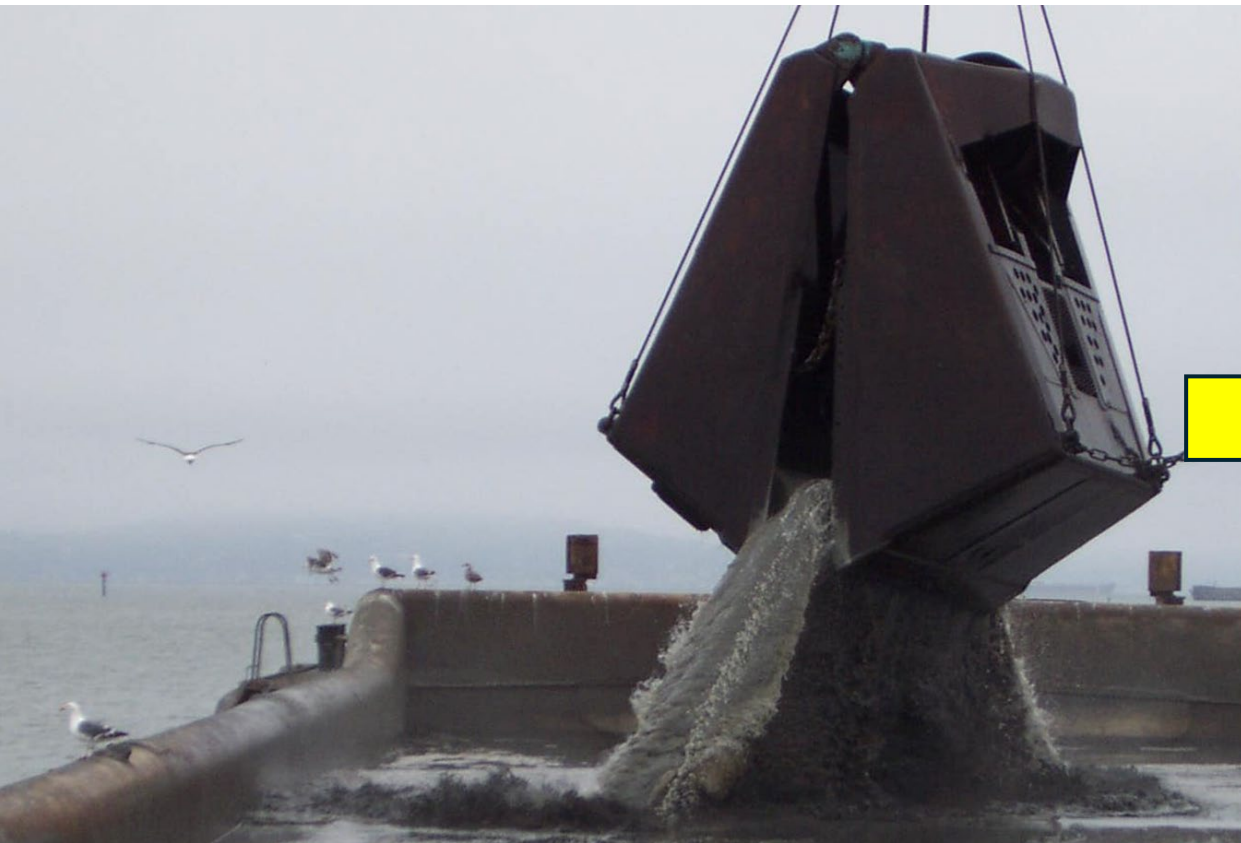
Sediment dredged from Bay, streams, channels
