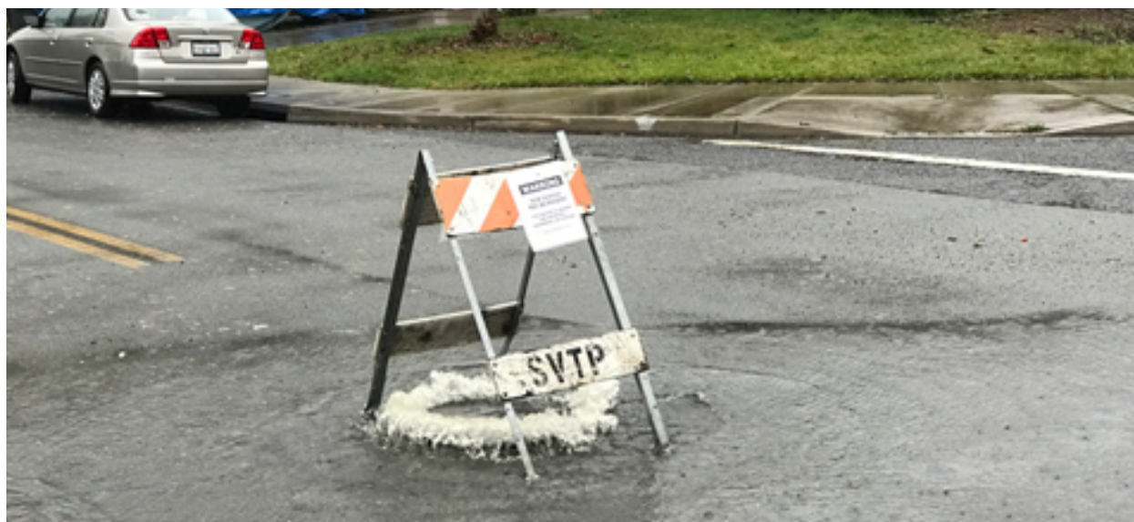
Sanitary Sewer Overflow (SSO) in The Springs neighborhood of Sonoma Valley.
