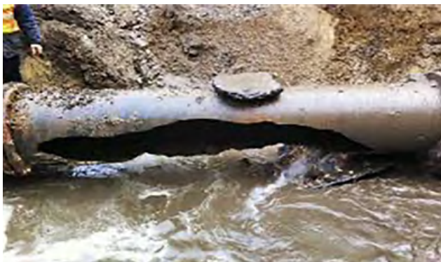
An example of a broken water main.
