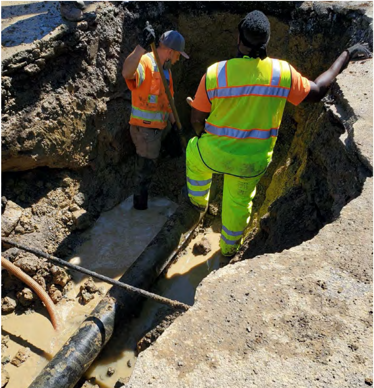
A broken pipe main in Marin City from Fall 2020 at the intersection of Phillips Drive and Drake Avenue. The break closed down a church and a school for a week as water overflowed.
