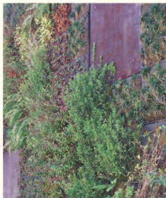
Green walls like this one at a motel in Portland, Oregon can slow and filter runoff from roofs. Photo by Lisa Owens Viani.
