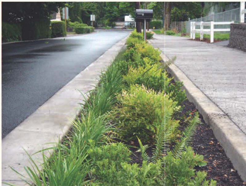
This residential street in Milwaukie, Oregon has no curbs, just a concrete border. Polluted runoff sheets off the road into the planter where it is filtered. Photo courtesy of Kevin Robert Perry.
