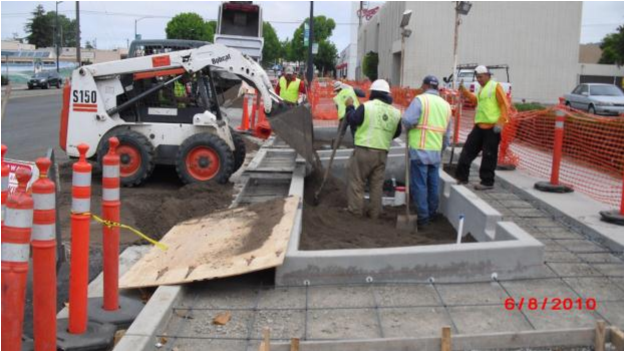
12 Filling rain garden cells with amended soils (native soils with organic matter), Eureka site.
